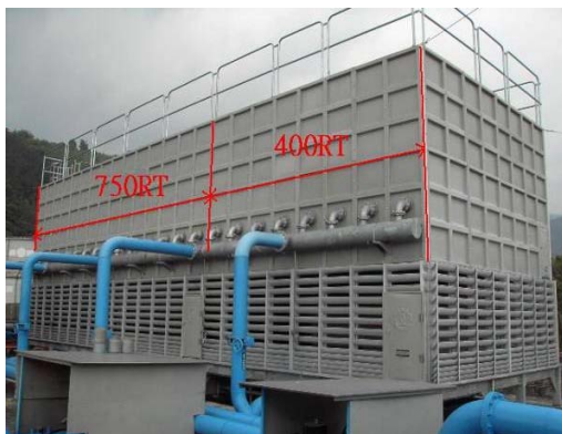
Fig. 3a: Fanless cooling tower appearance
