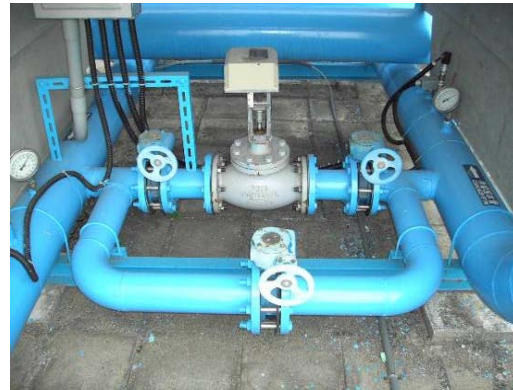
Fig. 5: Bypass pipe B
